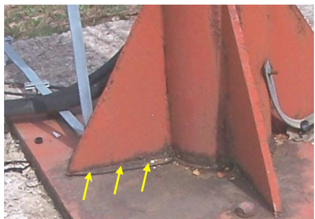
Fig. 7. Tensile crack caused by corrosion
