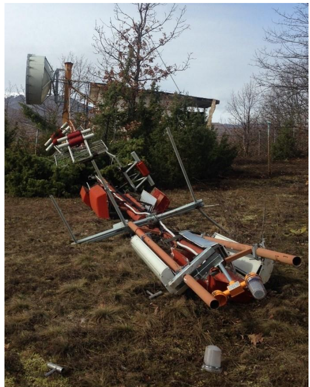
Fig. 3. Photo of the fallen mast segments
