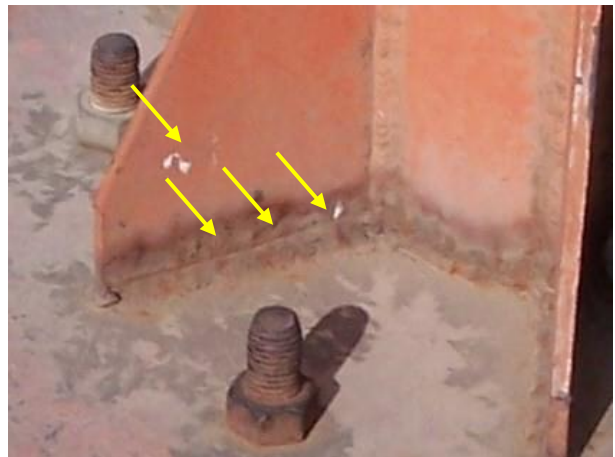
Fig. 6. Tensile stress crack caused by corrosion
