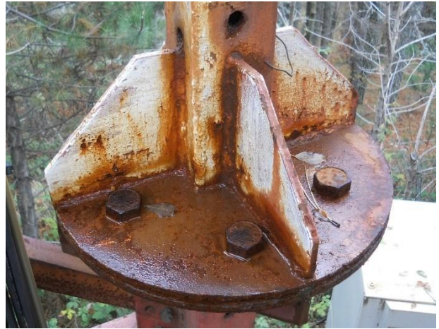
Fig. 5. Corrosion of the connecting flange
